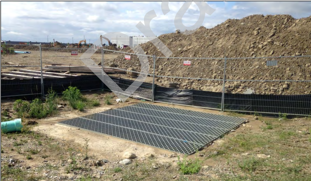
Photo 8: A galvanized steel grate reveals a portion of the lengthy underground piped watercourse enclosure that crosses and runs along the west side of Coleraine Drive.
