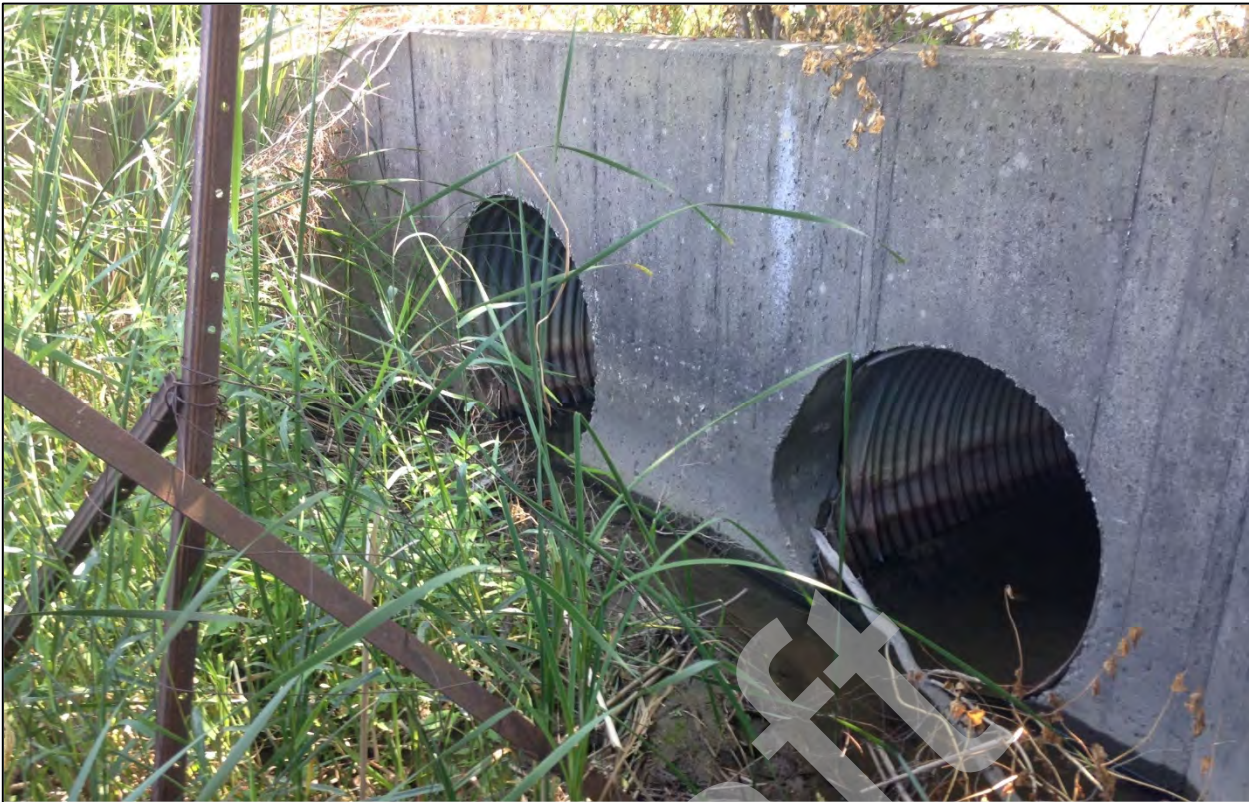
Photo 5: Upstream end of the double culvert outlet of SWMF #16. The culvert inverts drain the basin completely, with no permanent retention of ponded area within the basin.
