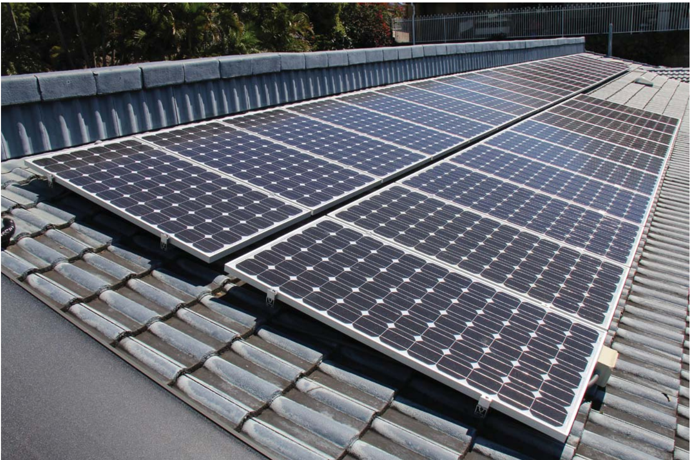
Figure 51: Rooftop Solar Panels
