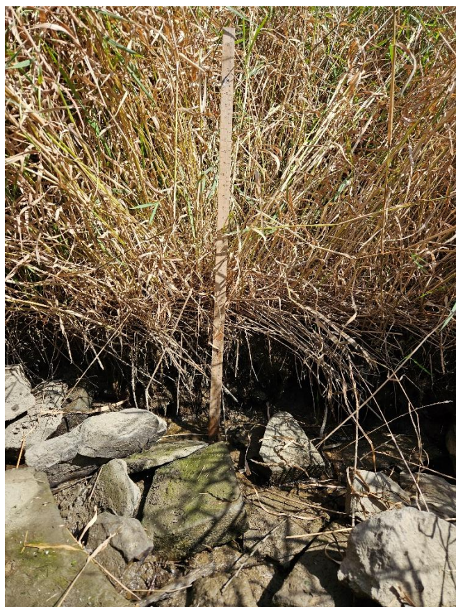
Photo 6. View of Salt Creek channel bank upstream from Mayfield Road. Photo taken on September 17, 2025.
