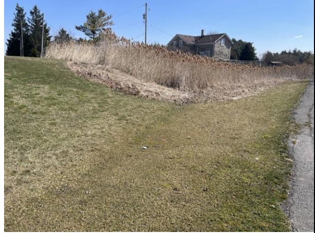
Photo 26 – H24-S1, golf course path depression looking downstream. (2024/03/27)
