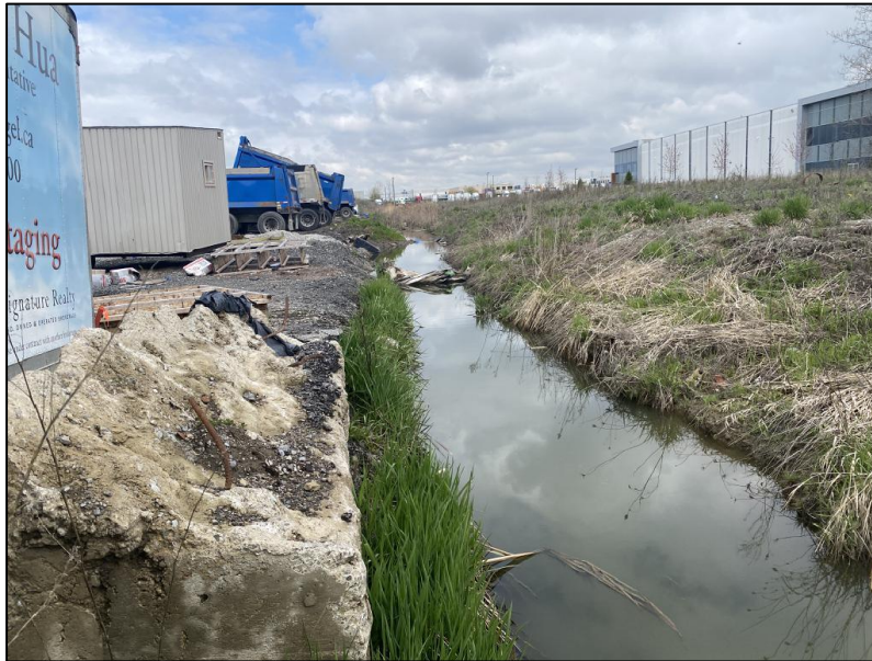
Photo 1: Concrete, fill and truck parking along the top of the west bank (photo taken facing upstream, north, May 2023).
