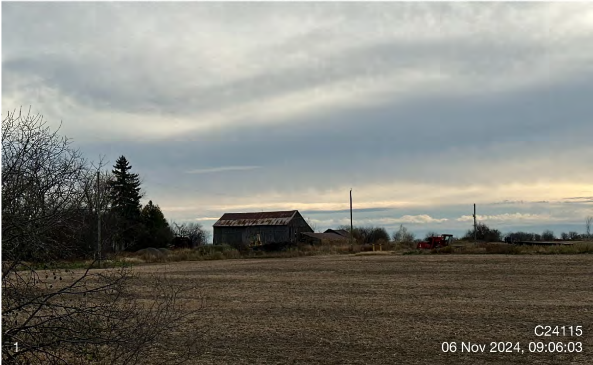
Photo 1: Operation #1 – Remnant farm, wooden bank barn in poor condition, missing boards.
