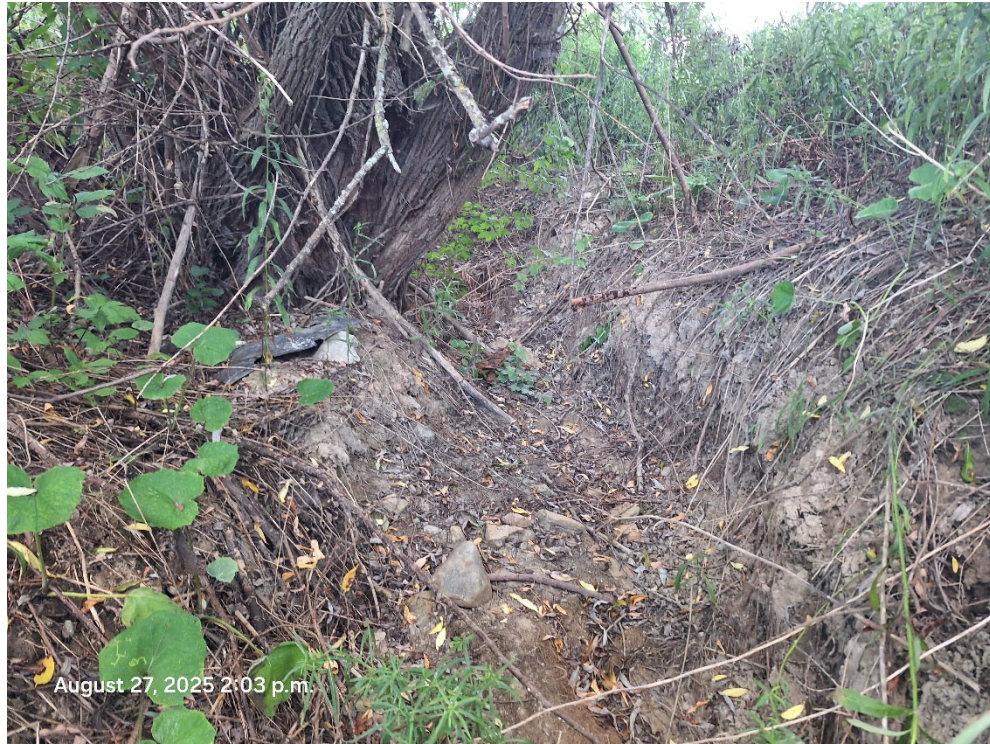
The downstream extent of the reach was defined adjacent to a tree, with local scour on both banks and exposed roots.
