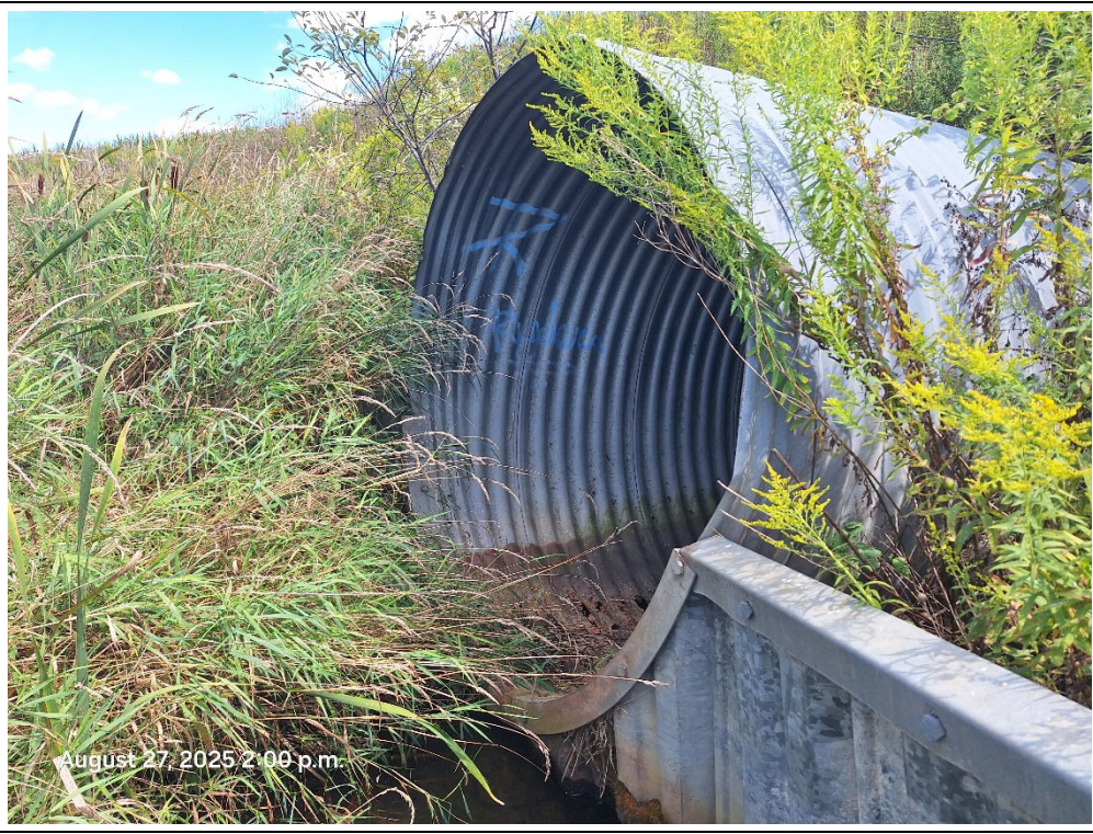
The culvert crossing Columbia Way was positioned at the confluence of two reaches, was perched above the channel bed, and was in disrepair.
