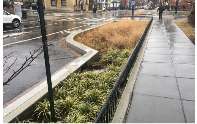
Bio retention swale for stormwater management
