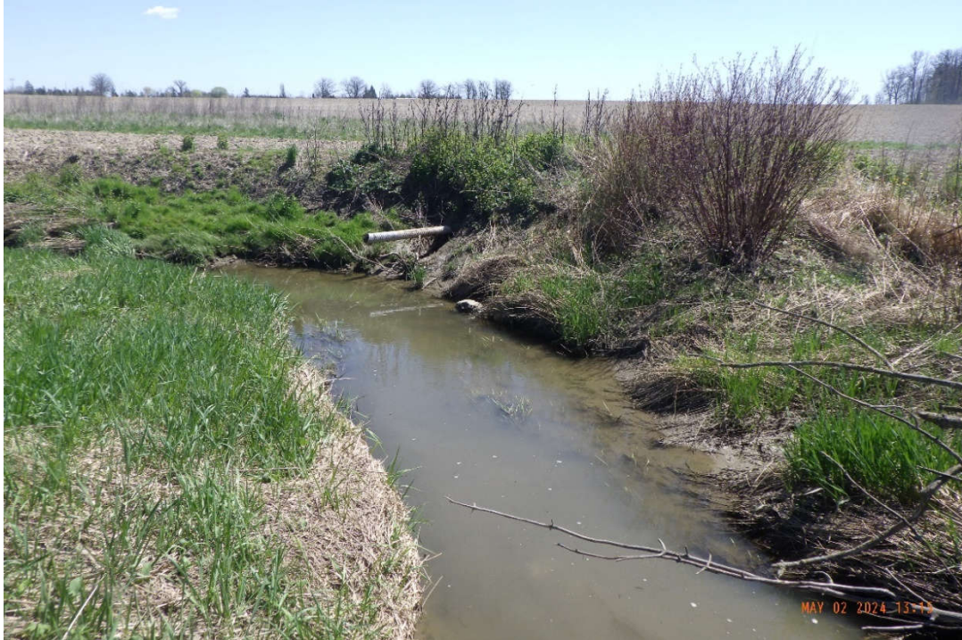
An exposed tile drain that was previously buried was observed at an outer bank of a meander bend and was in poor condition.
