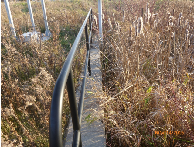
Figure 3.2 Overgrown Forebay Inlet – Looking West
