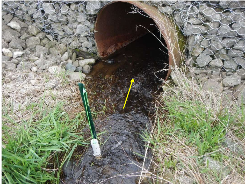
Photo taken facing downstream towards the Mayfield Road culvert after a 21.59 mm rain event.
