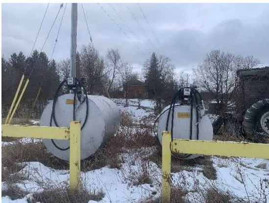
Picture 11: View of the two (2) diesel fuel ASTs (PCA-7) located west adjacent to Barn 2.
