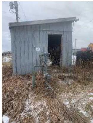
Picture 15: View of the natural gas connection to the utility shed, located in the central portion of the farm.
