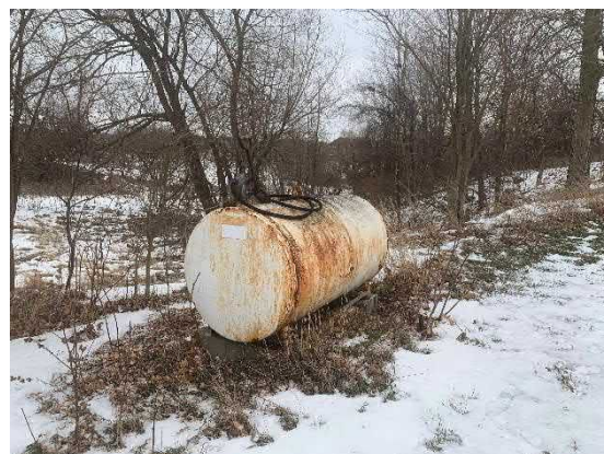
Picture 6: View of the 1345-litre gasoline AST (PCA-6) located to the west of Quonset Hut 1.
