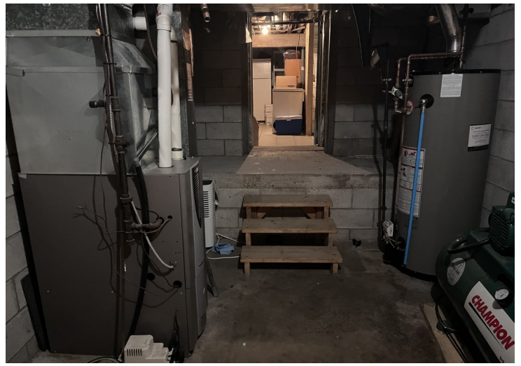
Photo 8: View of furnaces located in basement.
