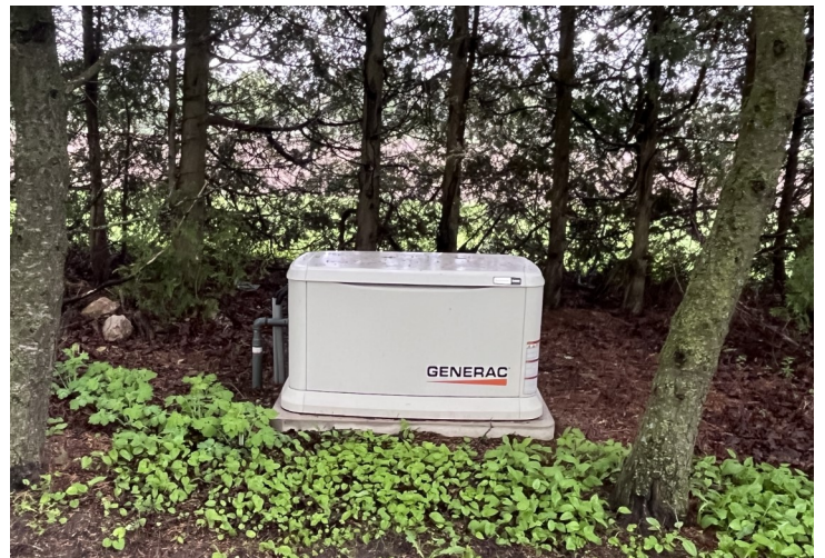
Photo 10: Natural gas fueled backup generator.
