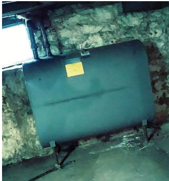
Photo 2 – View of the fuel oil AST located in the basement of Building #1.
