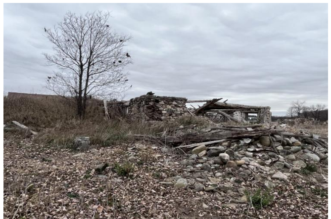
Photo 6: View of one of two previous buildings (Building 2) that has been demolished, located 15 m south of the current building on Site, fill pile containing stones and wood debris is located west of the foundation, facing east.
