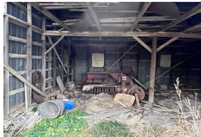
Photo 5: Interior view of Building 2 (scraps of lumber and metal, hay baling equipment), facing north.
