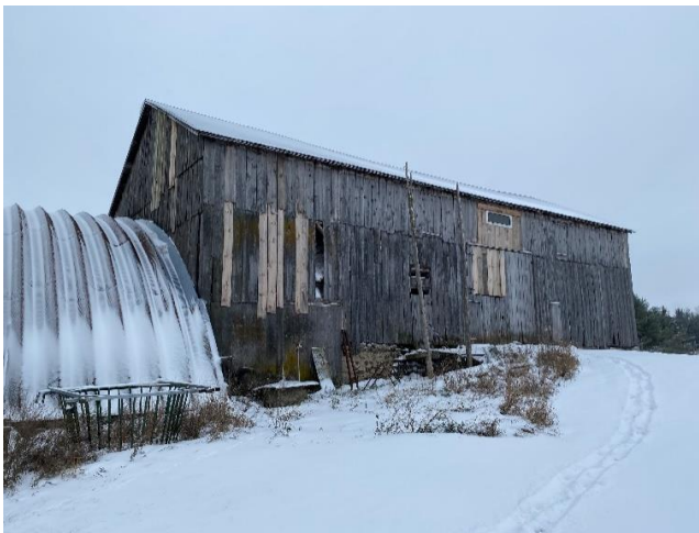
Plate 23: Oblique view of west elevation and steel Quonset addition of Barn No. 1.
