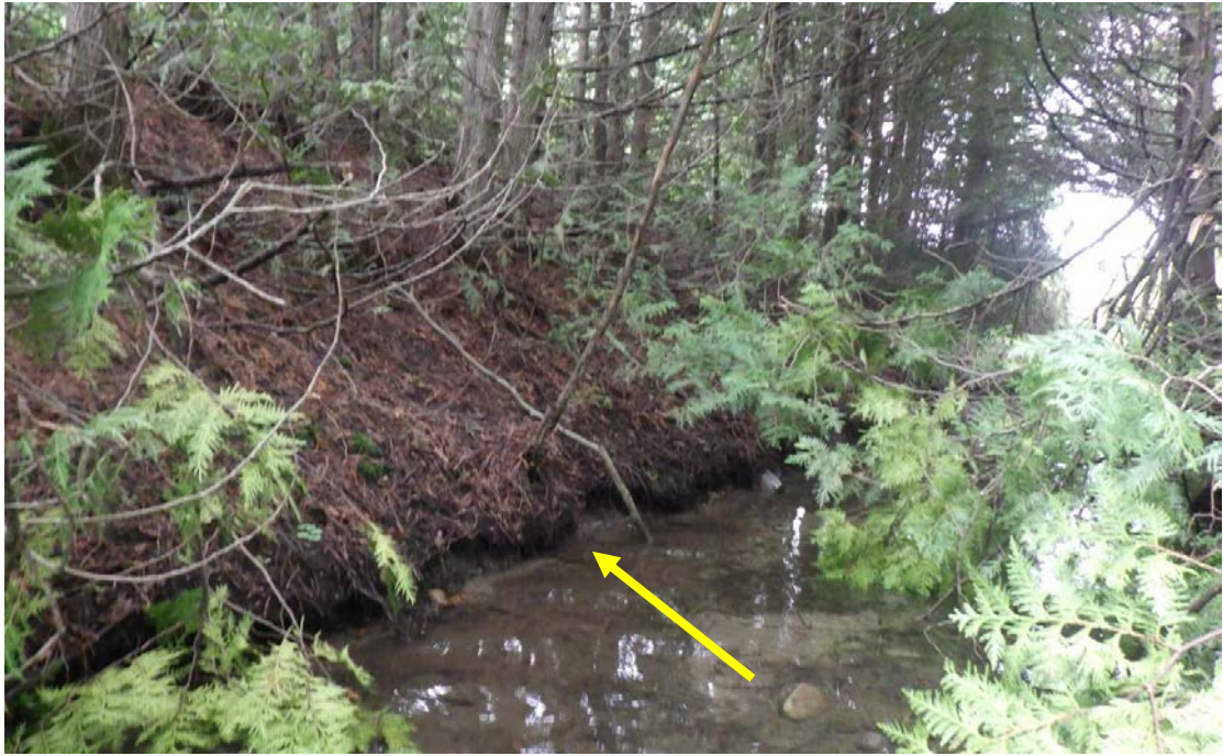
East Ponds Outlet Channel – facing downstream. Undercutting was observed along the left bank.
