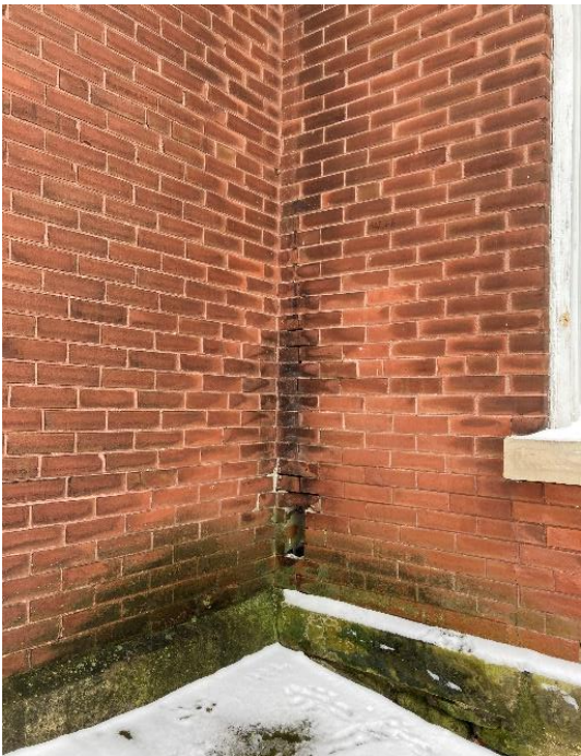
Plate 26: Location of former downspout on east elevation
