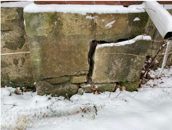
Plate 22: Deterioration in the foundation of the west chimney on the west elevation
