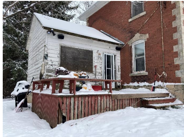
Plate 31: East elevation with former external chimney visible on original main block (highlighted in yellow)
