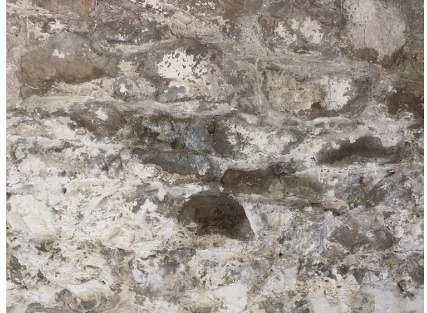
Plate 33: Parged stone foundation
