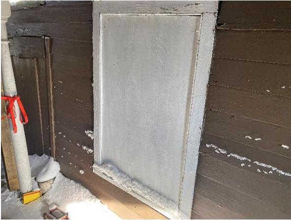
Plate 80: Framed window opening between frame and plywood addition to storage room/summer kitchen
