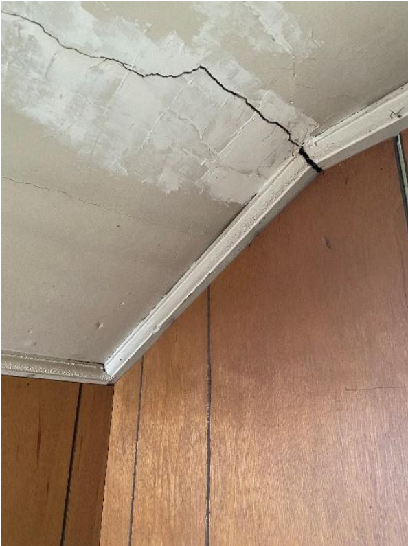
Plate 53: Cracks and repairs of southeast room
