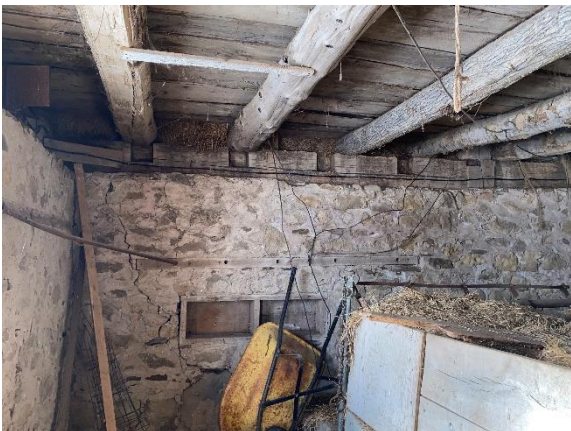
Plate 97: South barn interior, redundant mortices visible along sill
