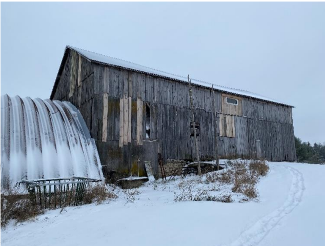
Plate 23: Oblique view of west elevation and steel Quonset addition of Barn No. 1.
