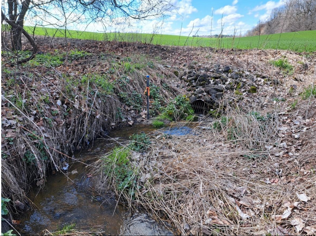
A tile drain with rip rap erosion protection was located at the upstream end of the reach. The riparian vegetation was fragmented in the upstream extent, where grasses were prevalent.
