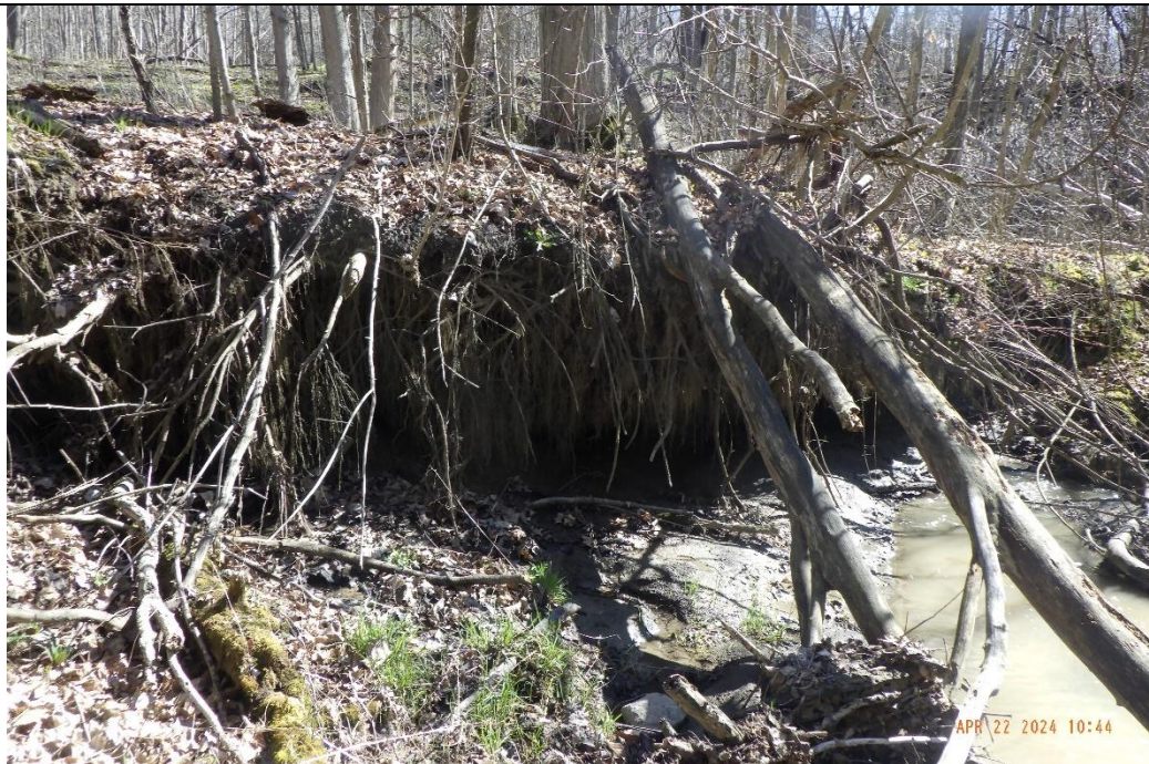
Erosion was found throughout the reach and undercuts measured up to 1.63 m.
