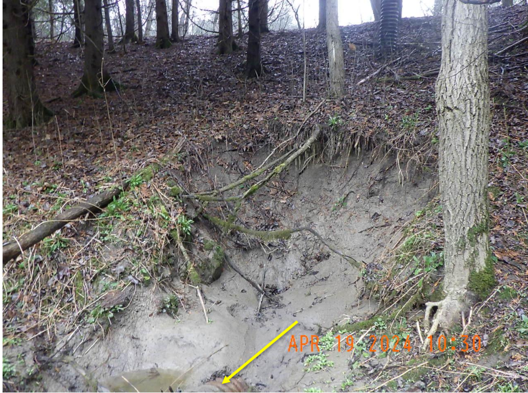
A mass failure had occurred at the downstream portion of the reach, exposing a pipe that was discharging into the channel.
