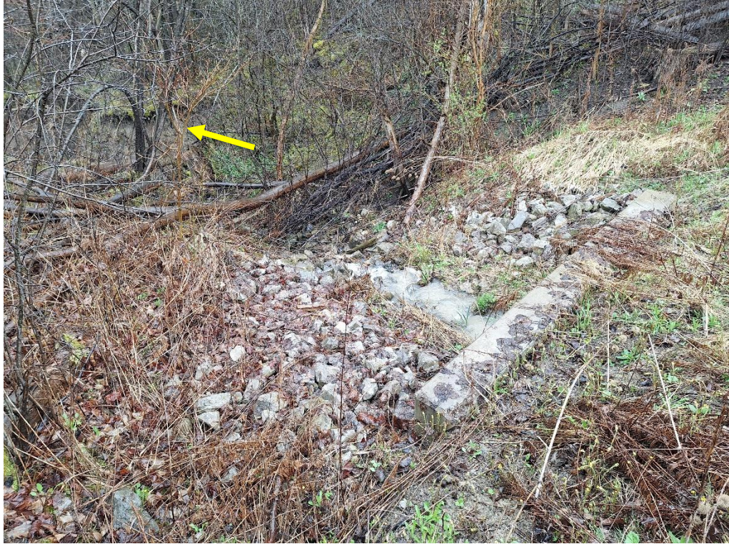
An outfall was present at the upstream extent of the reach at Duffy's Lane. Following the outfall the gradient changed significantly and erosion was observed immediately downstream (yellow arrow). Channel hardening was also present at this location.
