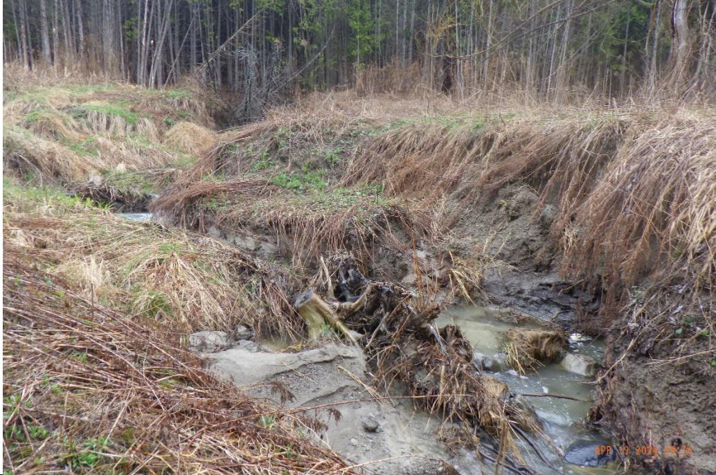
Multiple locations along the reach contained mass failures and fracture lines along the banks.
