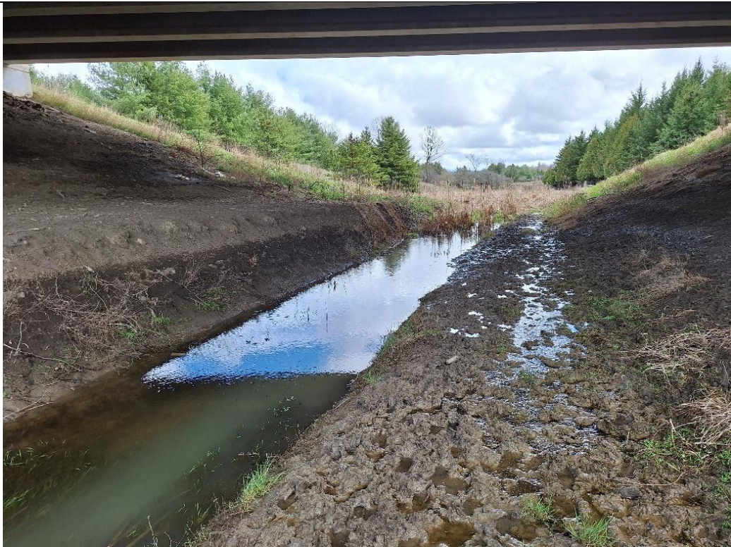
At the upstream extent of the reach the channel had been straightened under the bridge crossing.
