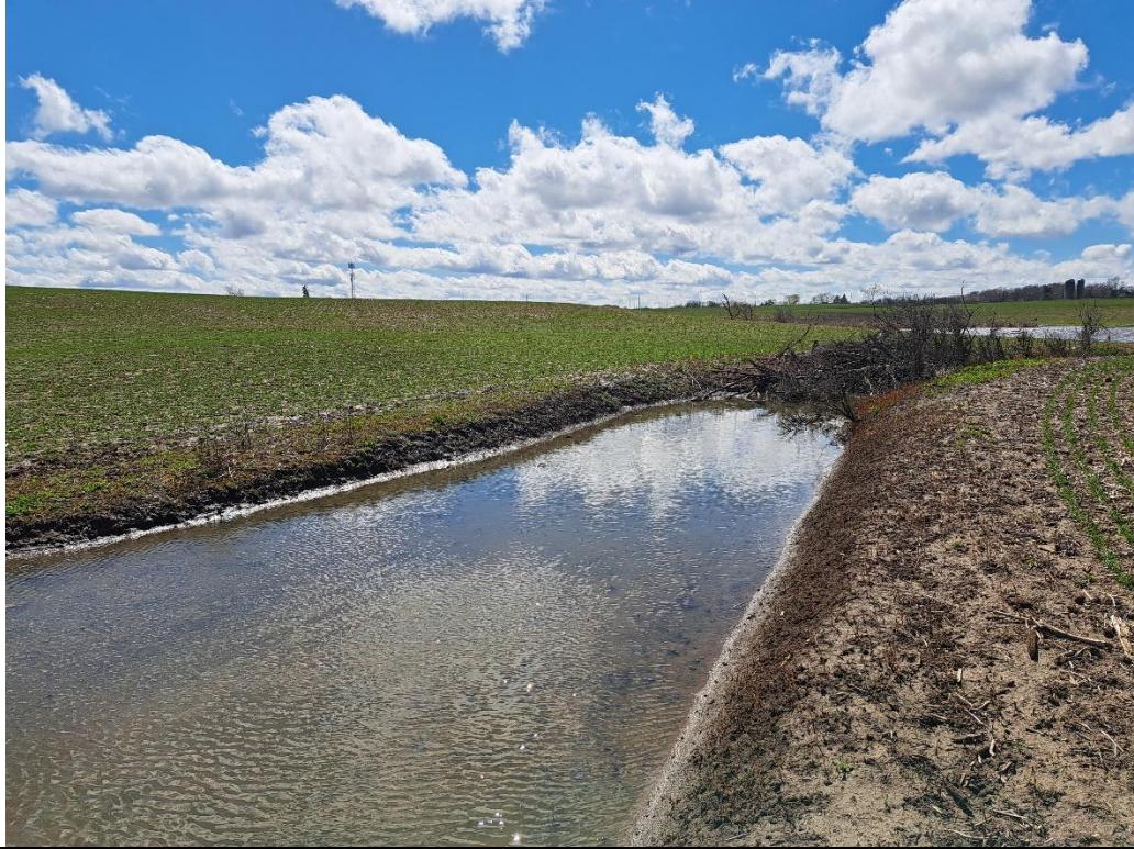
The bed and bank substrate were generally uniformly clay, silt, and sand.
