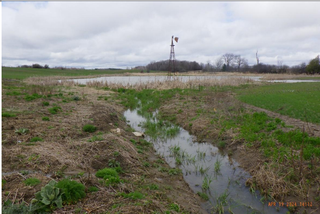
The pond outlet showed evidence of widening. Cattails and wetland vegetation were present at the outlet.
