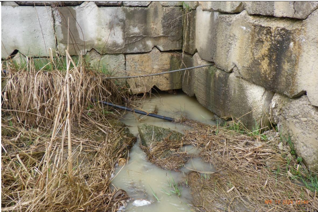
The downstream portion of the reach flowed under a concrete wall and was assumed to be piped. Due to access limitations, this was the furthest downstream observation collected along this reach.
