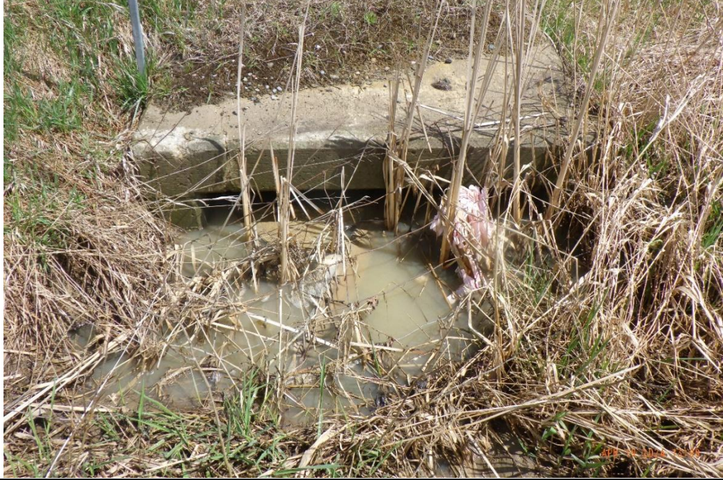
The rectangular concrete culvert at the road was silted and at approximately 75% capacity.
