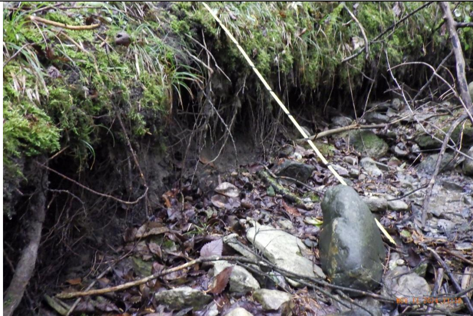
The channel was actively widening and contained undercuts measuring up to 0.69 m.
