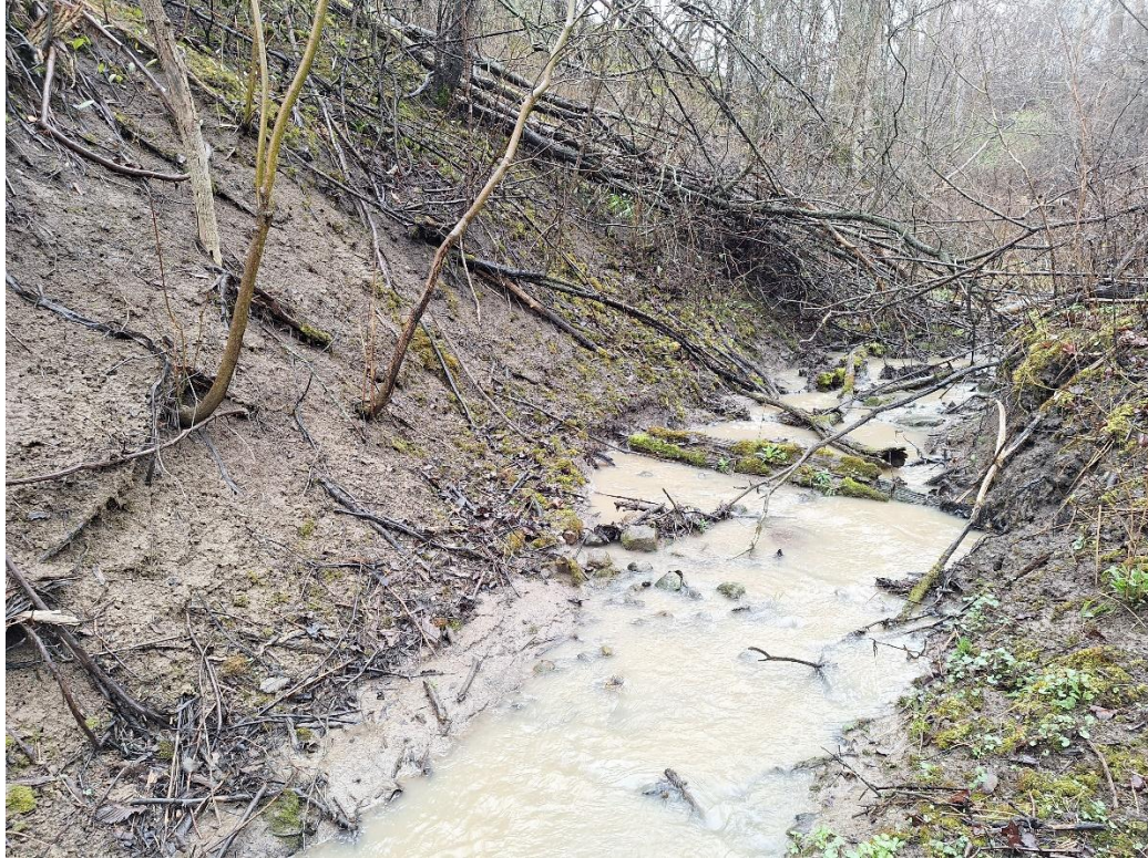
The channel bed substrate consisted of sand, gravel, and cobbles. The bank substrate was comprised of clay, silt and sand.
