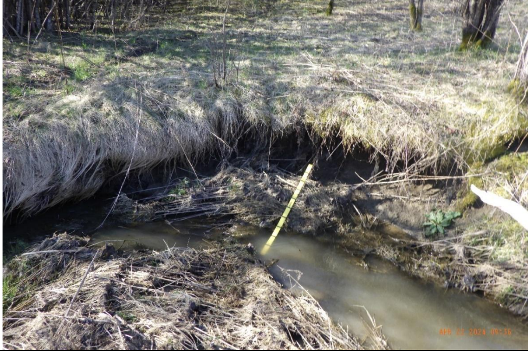
Erosion was observed throughout the reach. Meadow grasses covered the channel banks. Minor undercutting was observed.
