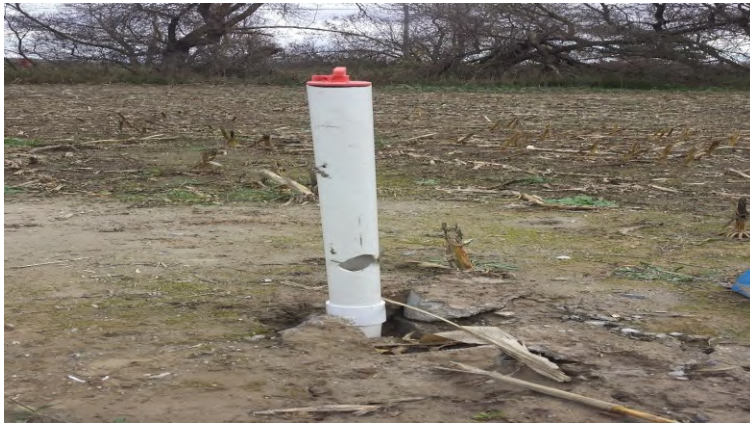
Photograph 2: View of the broken PVC pipe. A cut could be seen.
