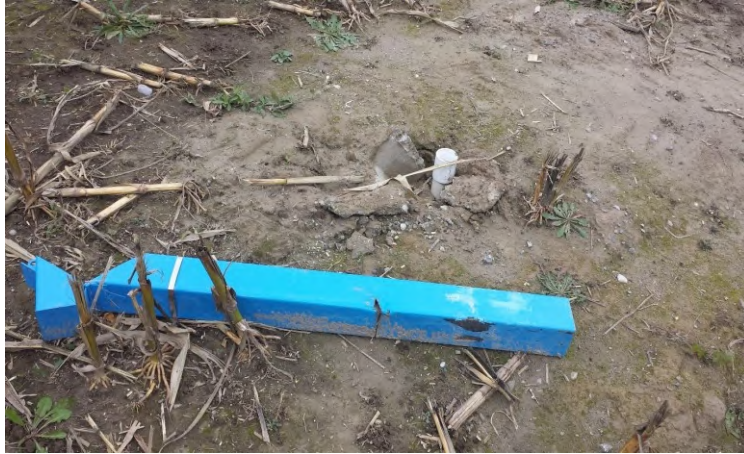
Photograph 1: View of the damaged monitoring well (MW8). The PVC pipe was broken and the protective casing was uprooted. A cut was noted in the protective steel casing.
