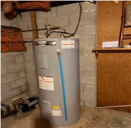
Picture 7: View of the water heater tank in basement of Phase I Property.
