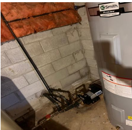
Picture 9: View of the well water pump in basement of Phase I Property.
