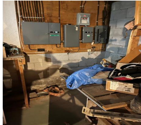
Picture 8: View of electrical panel in basement of Phase I Property.
