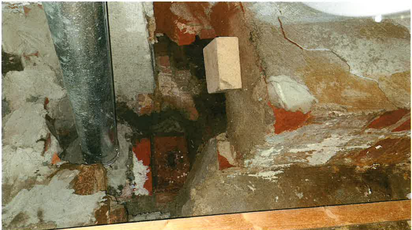
Former coal furnace located in the basement of the house at 14100 Humber Station Road
