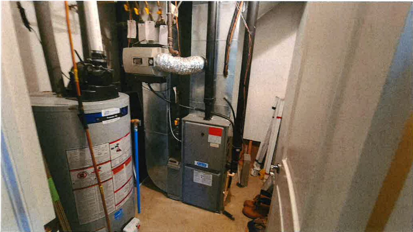
Utility room located in the basement of the house at 14166 Humber Station Road
