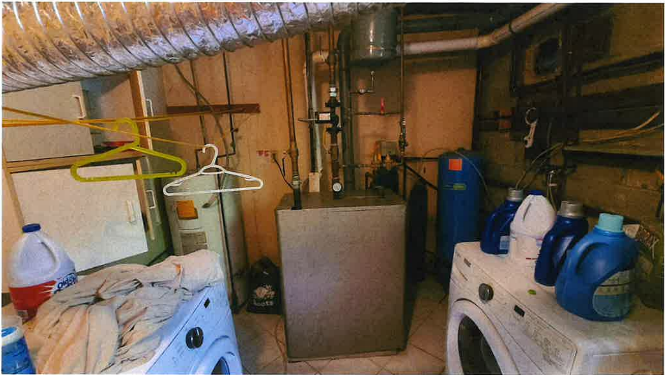
Utility room located in the basement of the house at 14196 Humber Station Road
