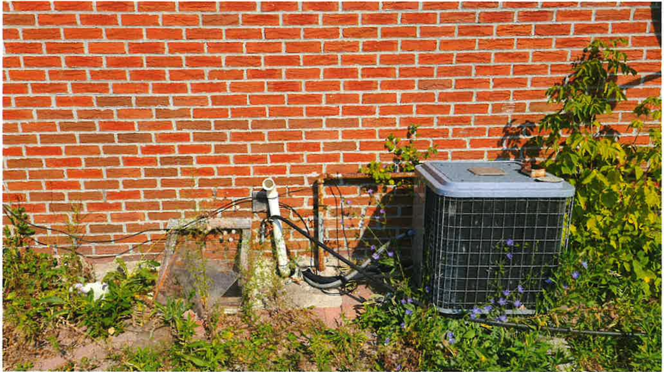
Former coal furnace chute on side of house at 14100 Humber Station Road (looking north)
