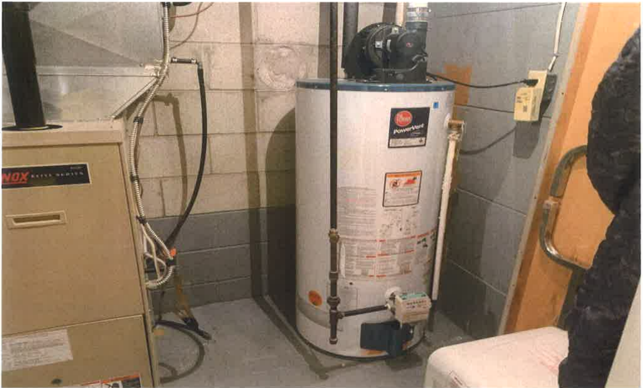
General view of hotwater tank in basement
