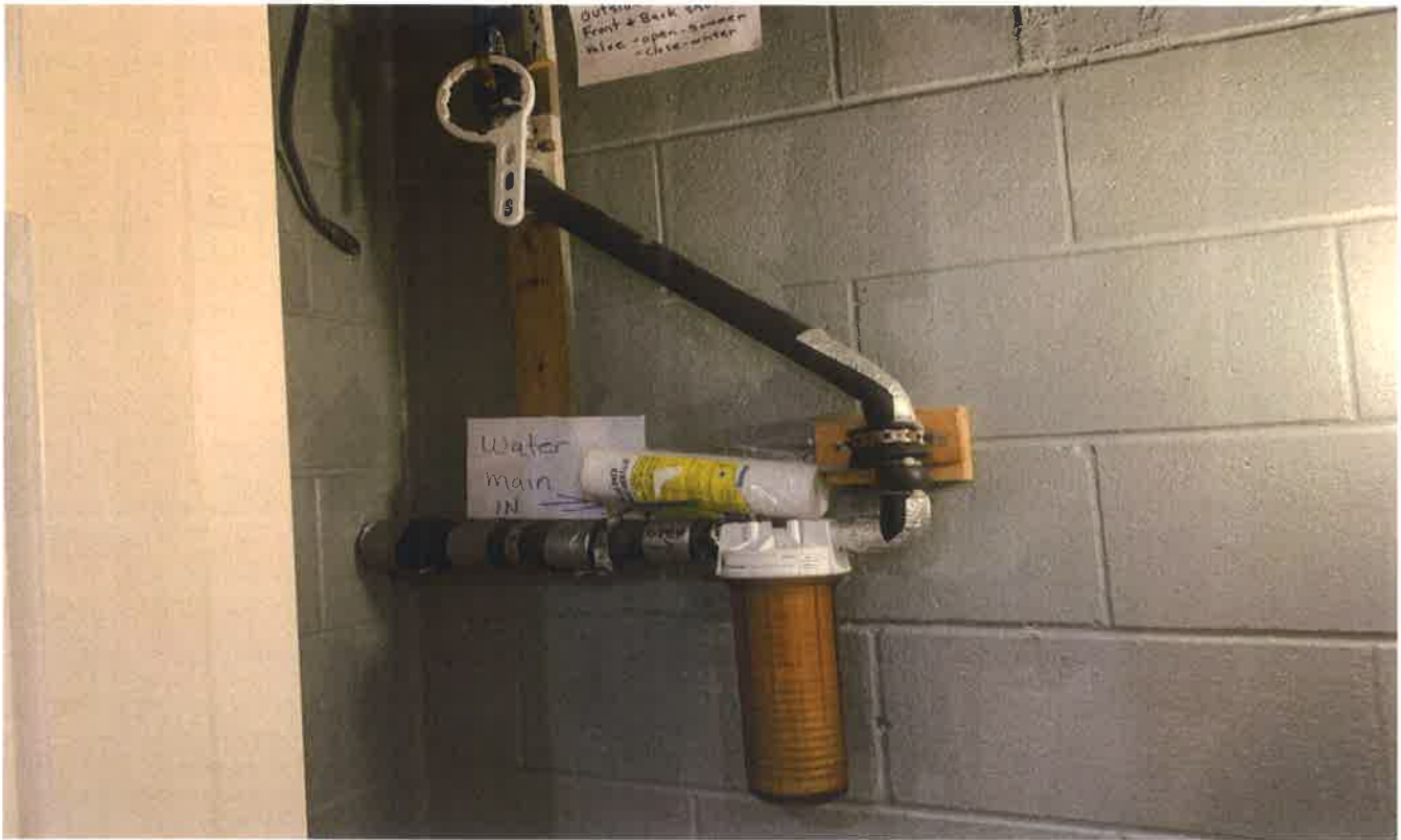
General view of water main in basement
