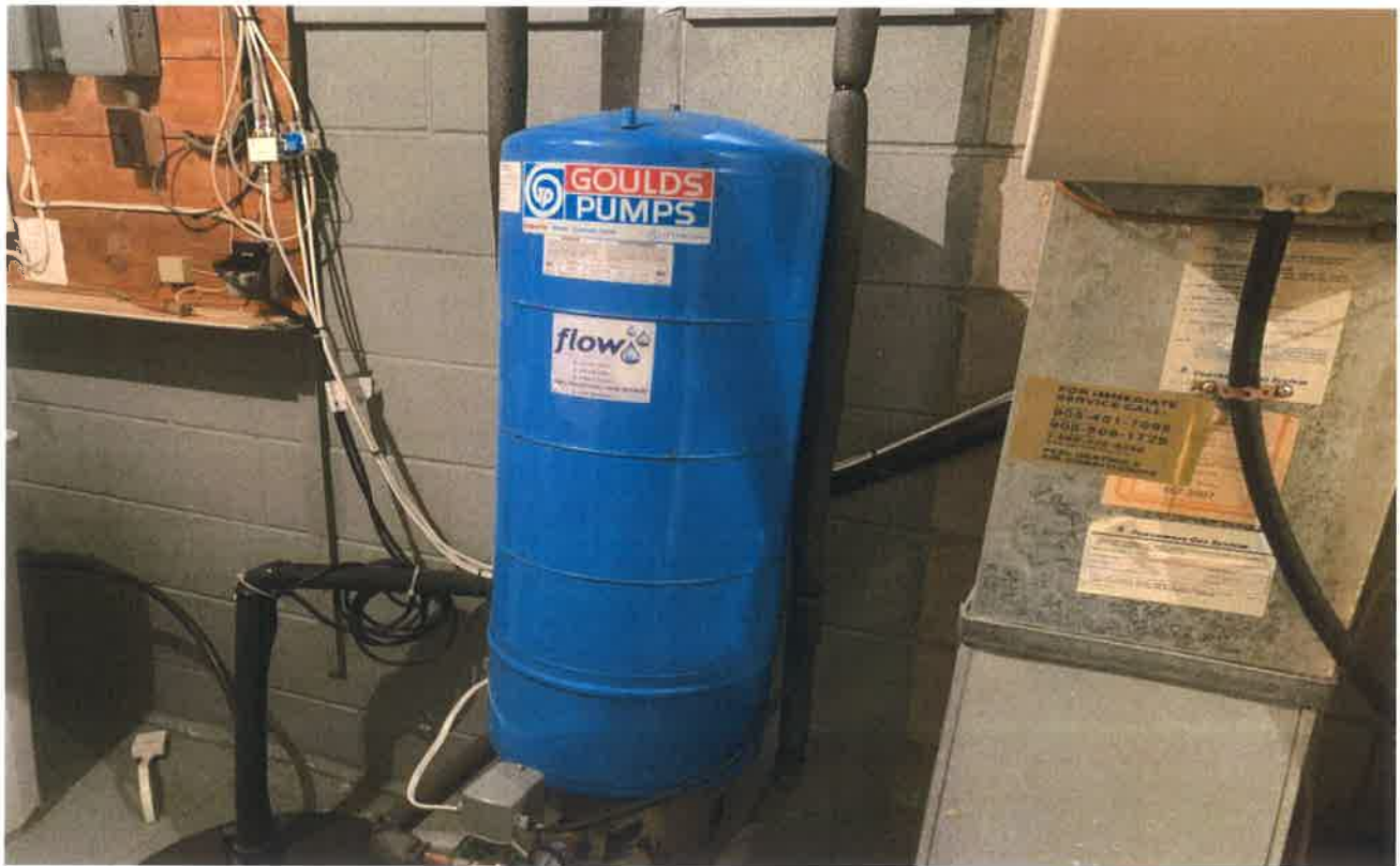
General view of water system tank in basement
