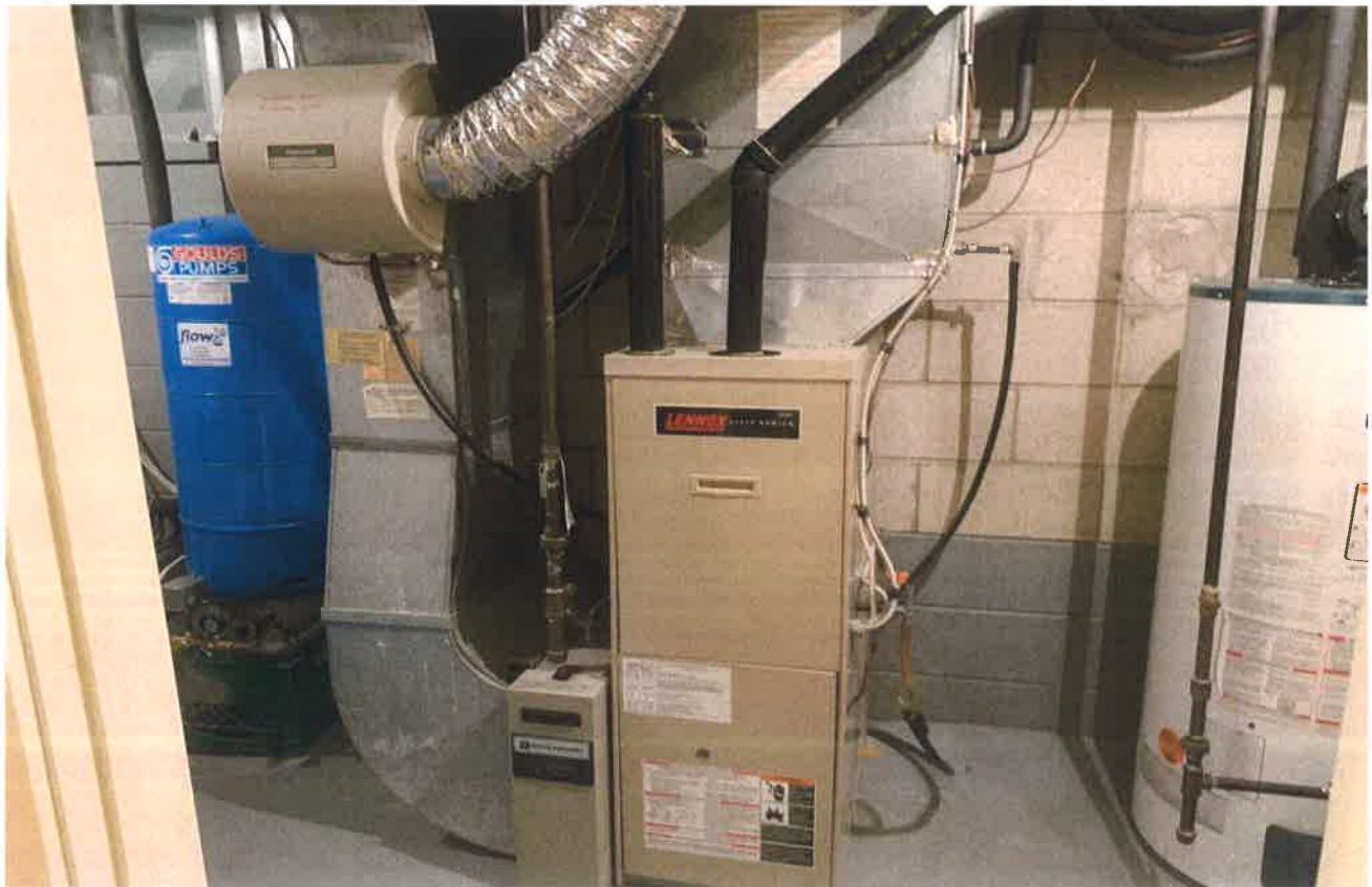
General view of furnace system in basement
