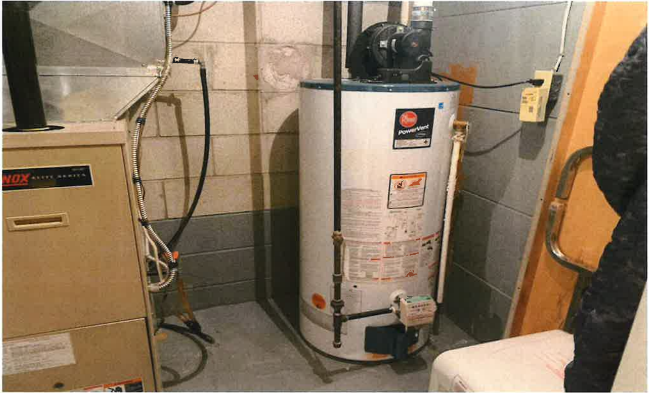
General view of hotwater tank in basement
