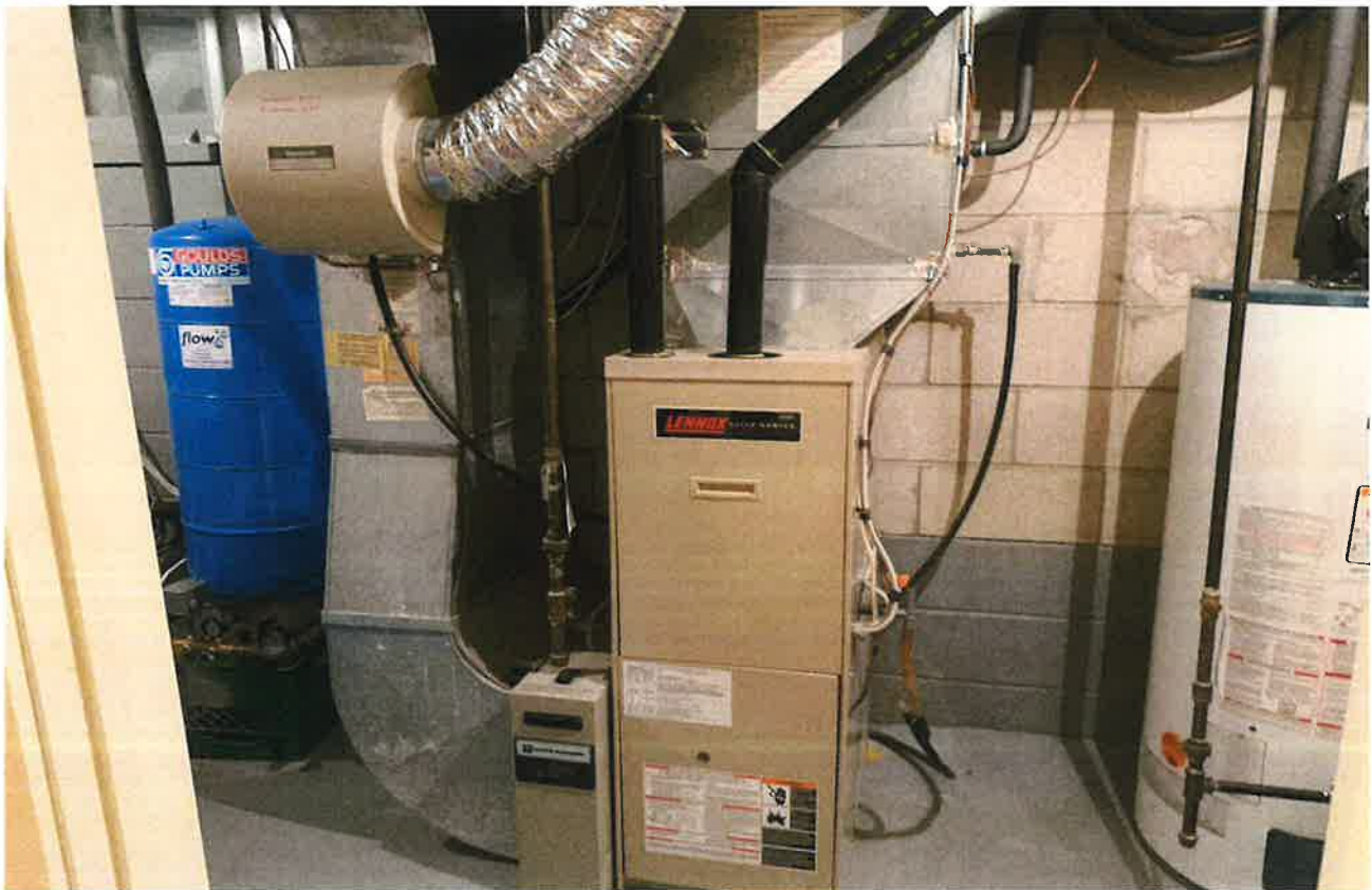
General view of furnace system in basement
