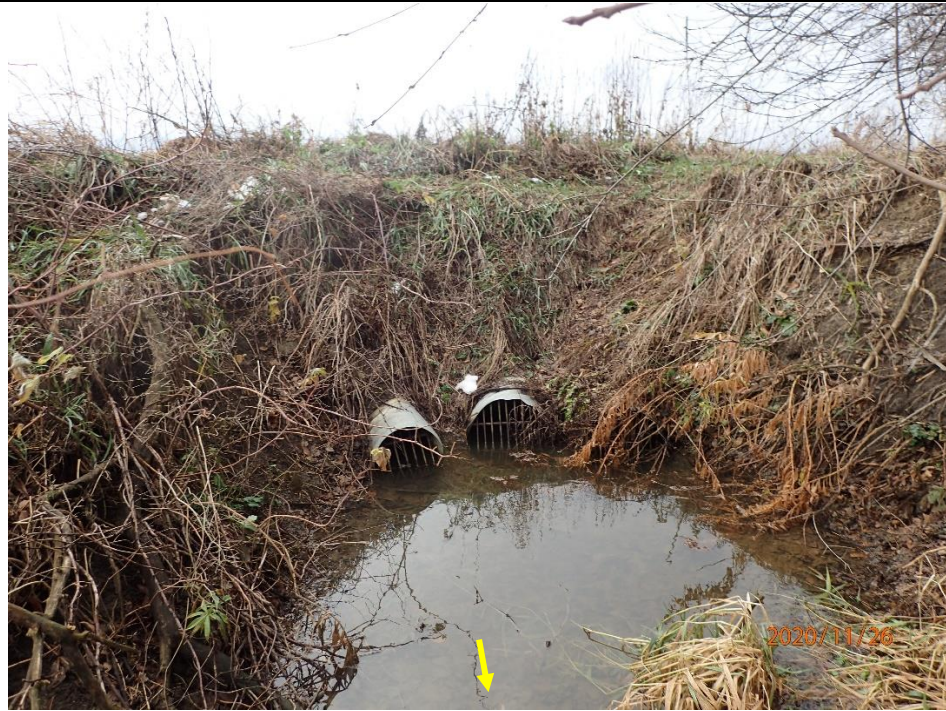
At the furthest upstream extent of the reach, tile drains were observed conveying flows beneath the agricultural field and into the watercourse. An enlarged scour pool was present immediately downstream from the tile drain outlets.
