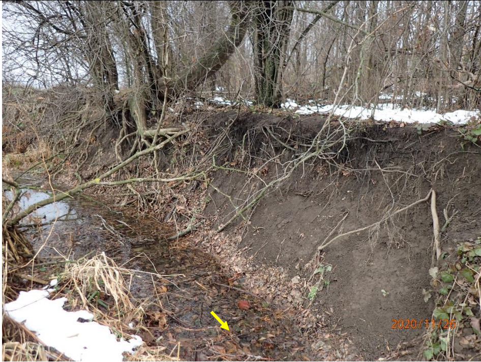
Photograph looking towards left bank (facing downstream). Valley wall contact was observed in this location, in addition to erosion scarring and exposed tree roots.
