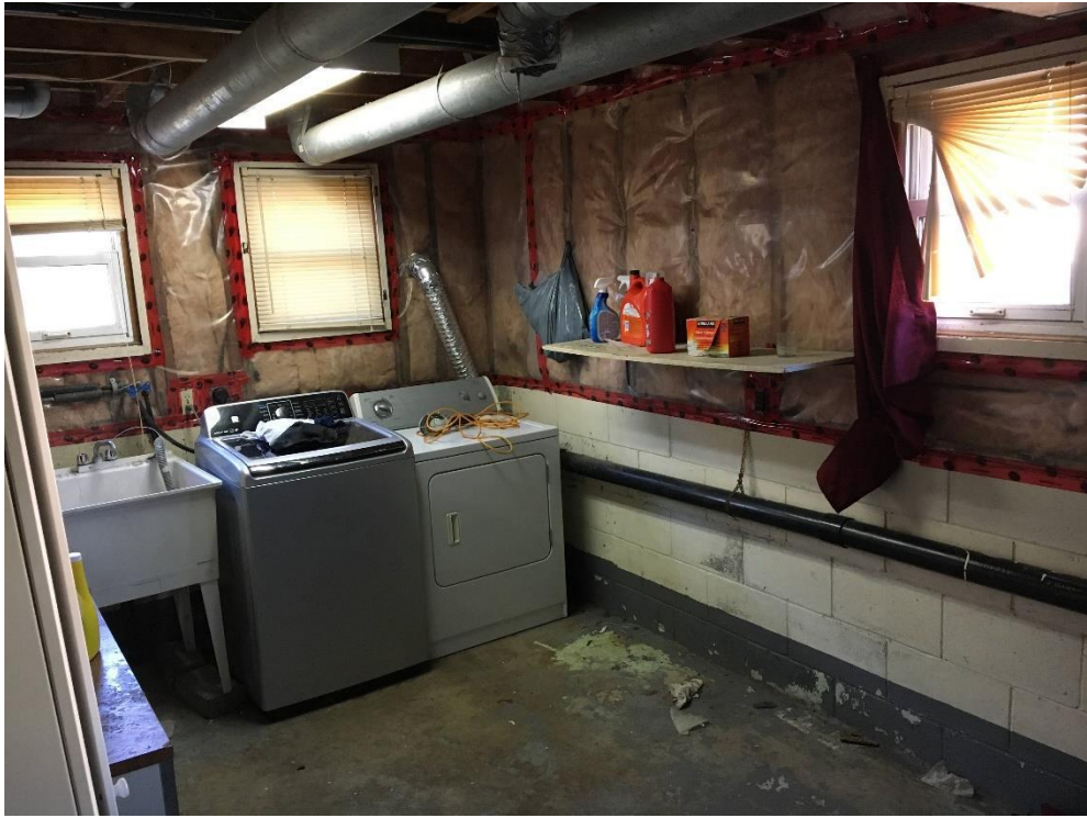
Photo 8: View of the laundry room near the northeast corner of the basement, looking northeast.
