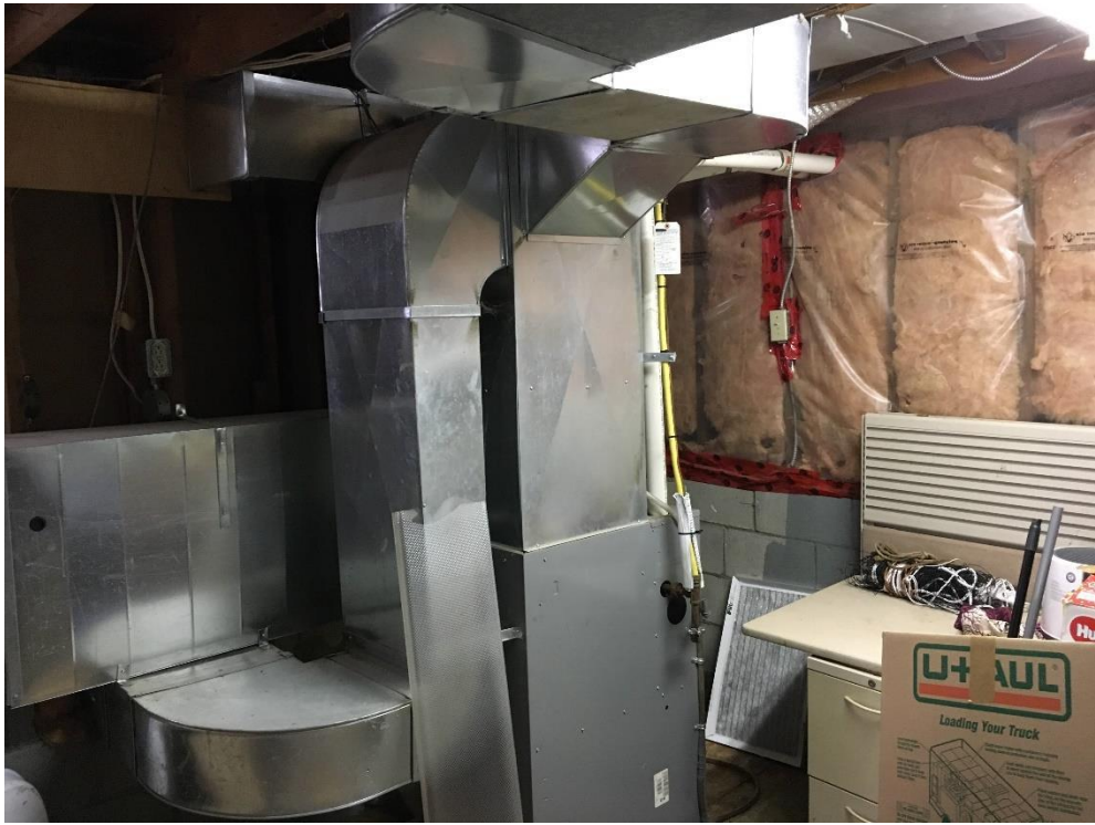
Photo 10: View of the gas furnace and fibreglass insulation near the central-western portion of the basement, looking southwest.
