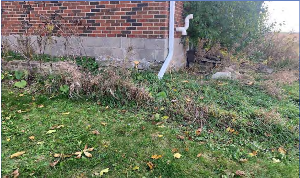
Photo 9: View of the brick siding, and the concrete foundation on top of the fieldstone foundation
