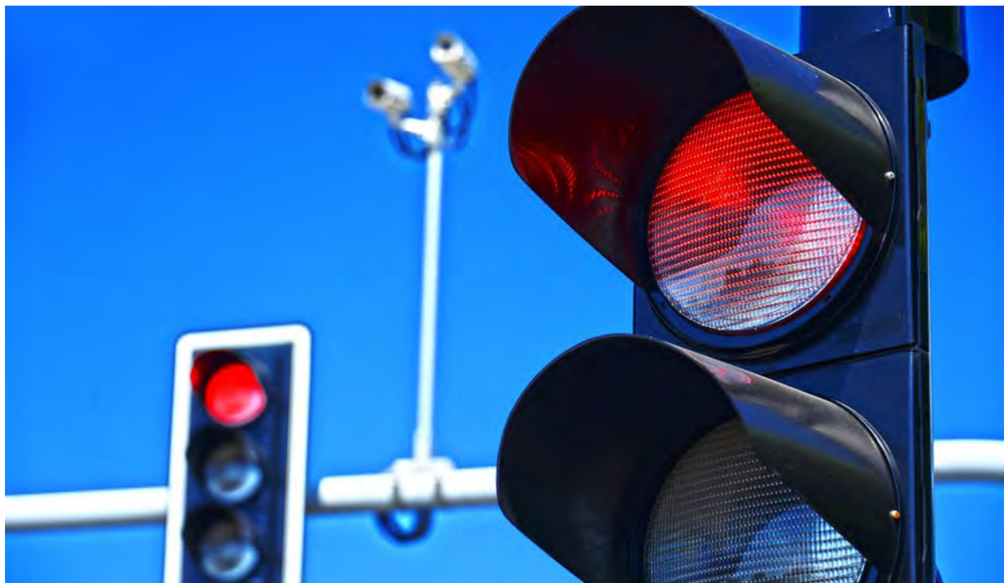
Smart Municipal Infrastructure
