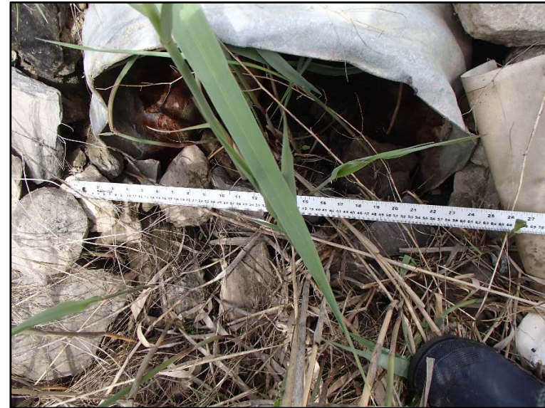
Photo 30: 2017-05-24, south end of culvert at D6 which crosses under the roadway between Highway 410 and Snelcrest Drive.
