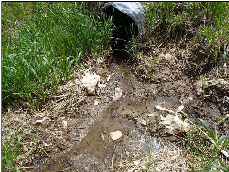
Photo 23: 2017-05-24, roadside drainage at D1 at north end of culvert under private driveway.
