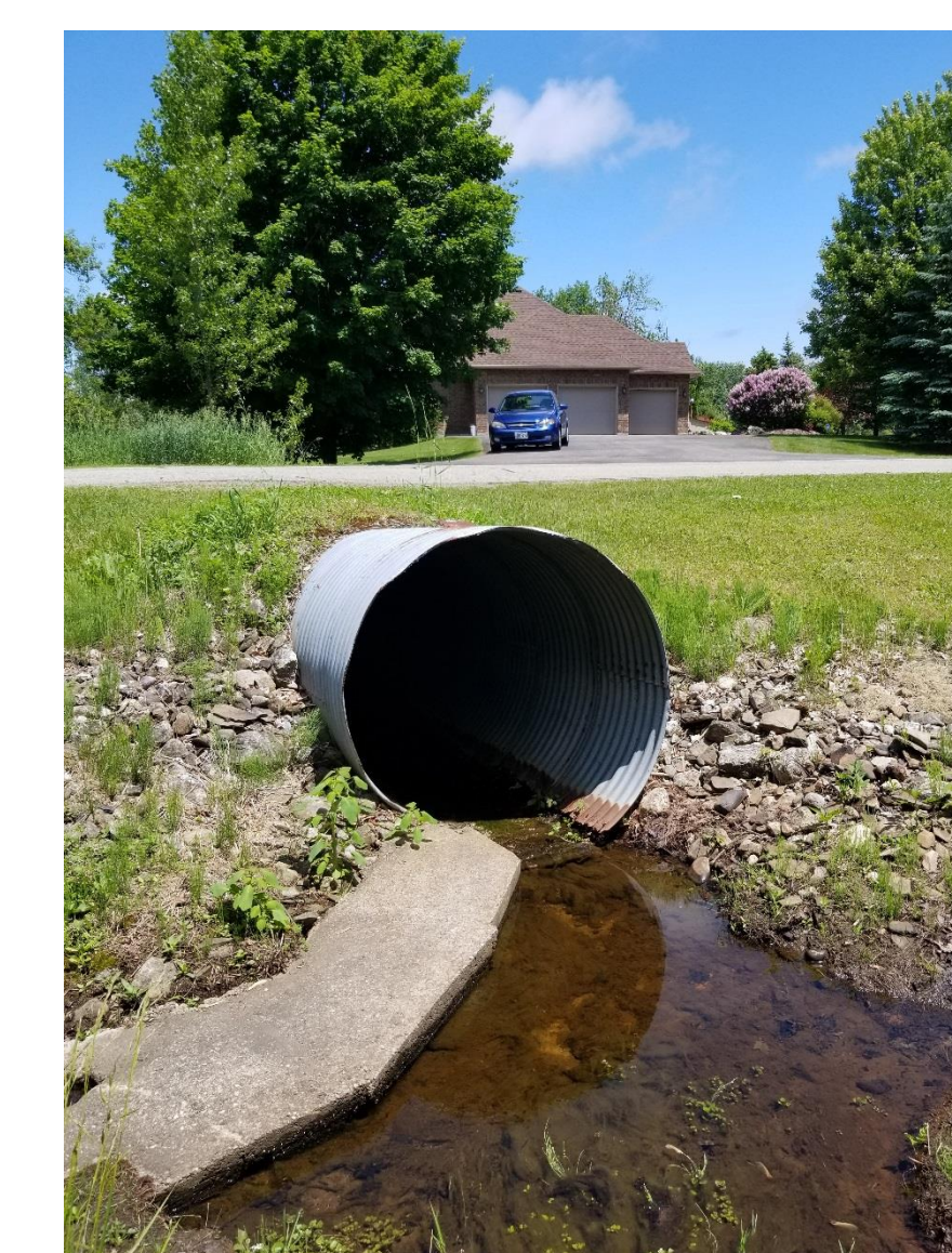
Large wooded debris in culvert (left). Bottom of culvert is rusted and may soon require replacement (right).
