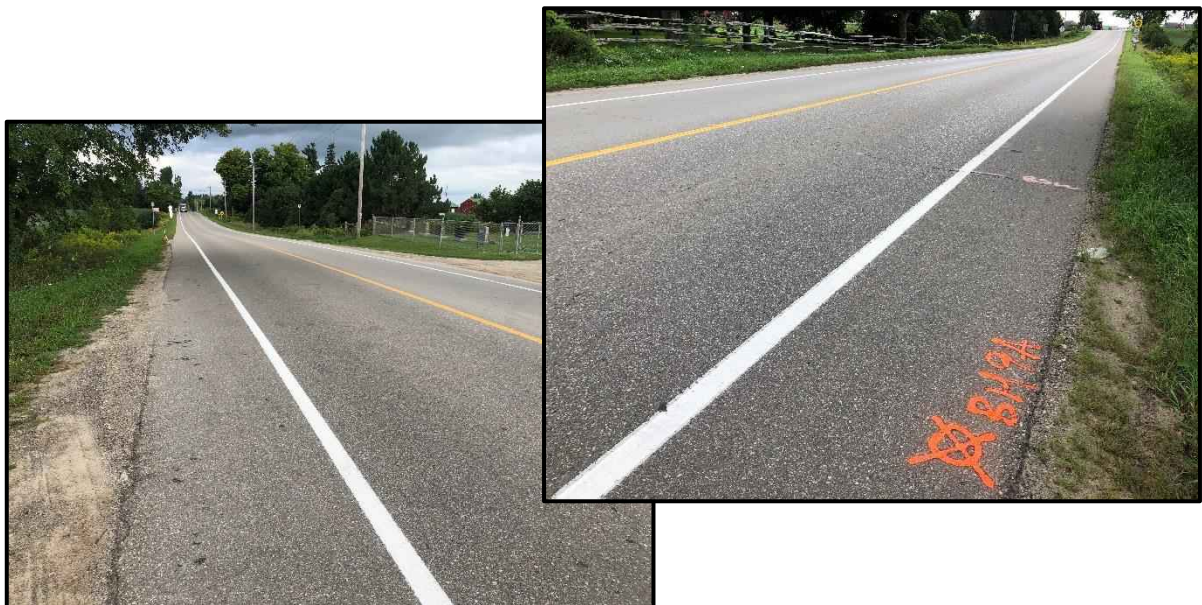
Figure 1: Overall Pavement Condition - Noting Local Transverse Cracking and Pavement Shoulder Edge Drop Off [GH 20180824]
