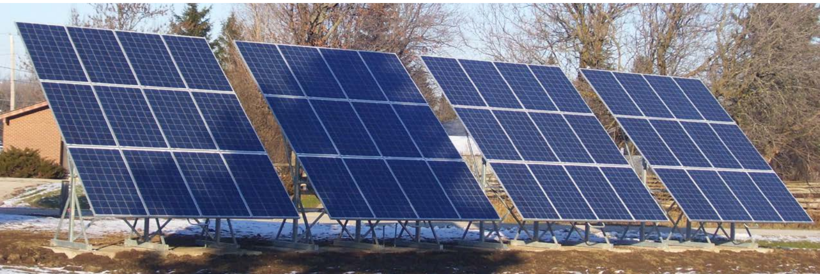
Photo: Town of Caledon solar installation.
