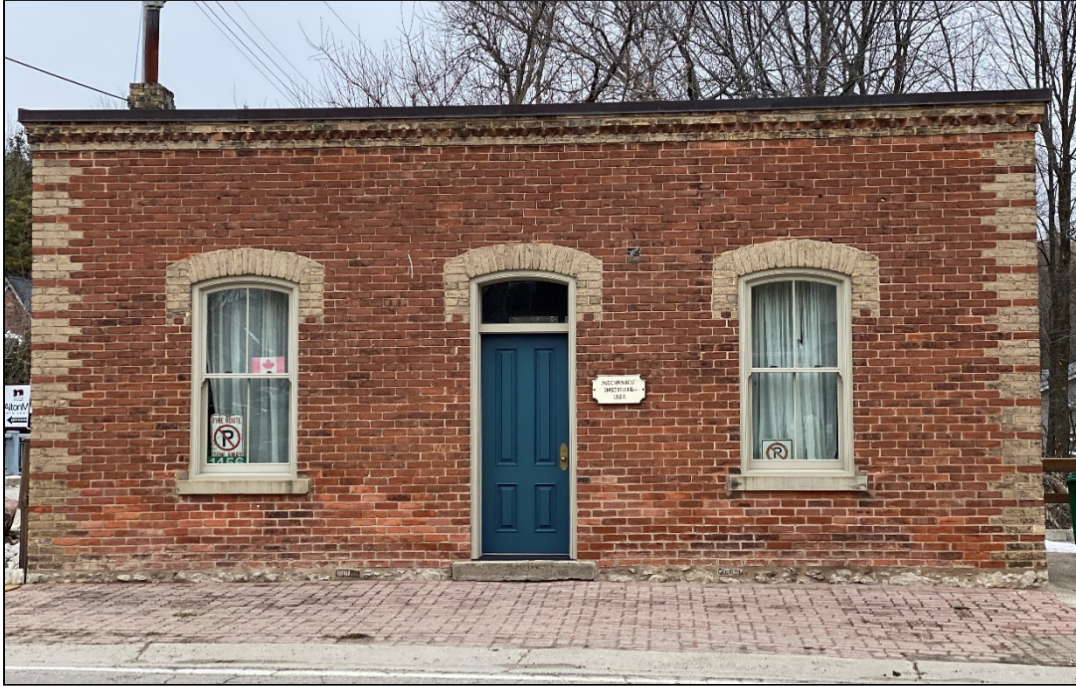
Image 1: Alton Mechanics Institute: repaired roof and flashing; repointed brickwork; replaced windows and front door
