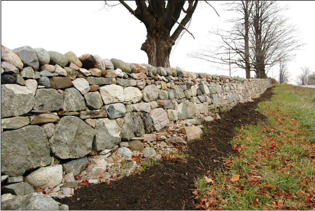
Image 11: Patullo-McDiarmid Dry Stone Wall: restored using existing stone and new cedar shakes.
