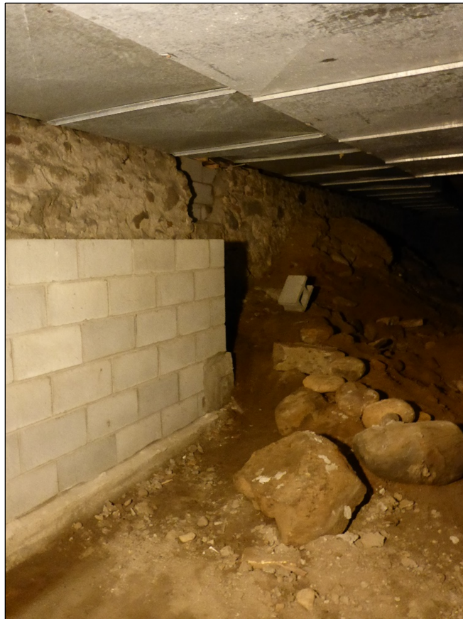
Image 6: Belfountain Village Church (17258 Old Main Street): emergency grant foundation repair
