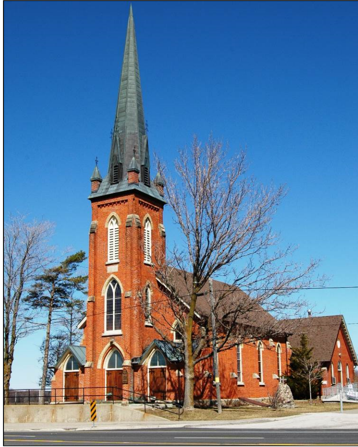
Image 9: Claude Presbyterian Church: repaired front gable fascia and soffits; painted exterior wood trim and exposed rafters in eaves
