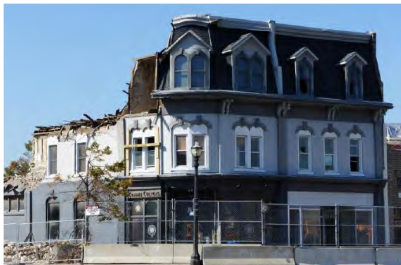
197. Catastrophic event, tornado damage, Goderich HCD, Ontario. (Source: www.ontariopics.com)
