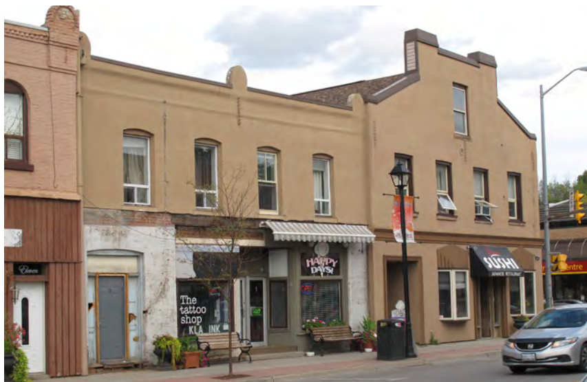
138. 5, 7 and 9 Queen Street North storefronts exposed following removal of modern cladding in August 2015, Bolton. (Source: Town of Caledon)
