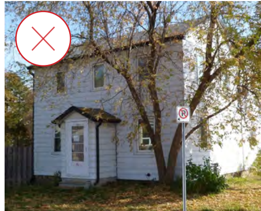
43. The size, proportions and texture of vinyl and aluminium siding are incompatible with the style of historic buildings in the District, 26 Mill Street (Source: ERA)
