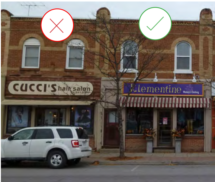
102. Original window openings and patterning have been maintained in new window design and installation at 19 Queen Street North (right) in contrast to poorly modified window openings on 23 Queen Street North (left), Bolton. (Source: ERA)
