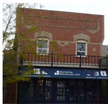
125. Flat roof concealed by parapet at 42 Queen Street North, Bolton. (Source: ERA)
