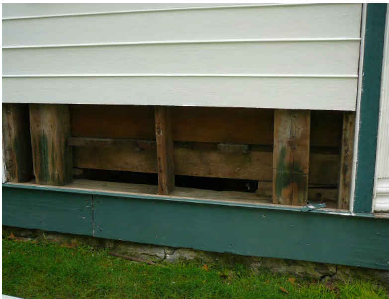
55. Investigate and document existing conditions and construction before repairing and replacing cladding. (Source: ERA)
