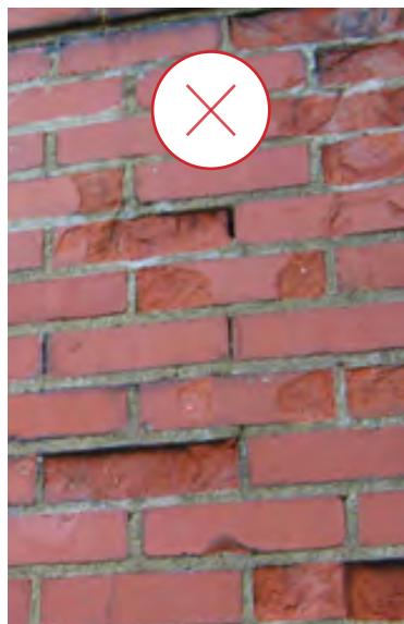
52. Spalling results from lack of maintenance and/or re-pointing with inappropriate hard mortar. (Source: ERA)
