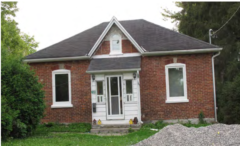
50. The removal of synthetic siding at 56 Nancy Street revealed the original brickwork and architectural detailing, Bolton. (Source: ERA)
