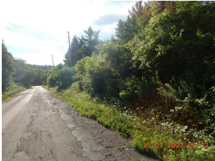
Photo 4: View of Glasgow Road condition, south side and facing towards Deer Valley Drive. July 26, 2022.
